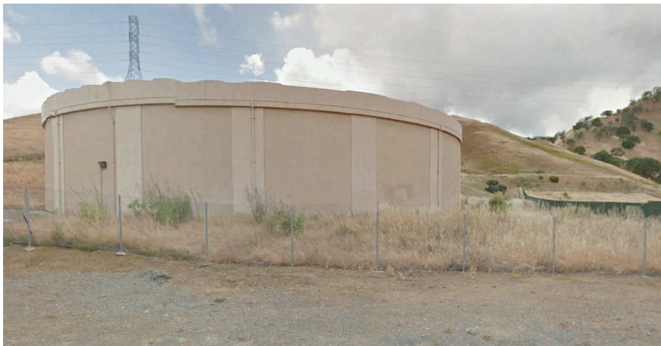
Figure C-10. Seismic Durability Assessment – The assessment will include the City’s water reservoirs such as Cambridge Reservoir shown above.
