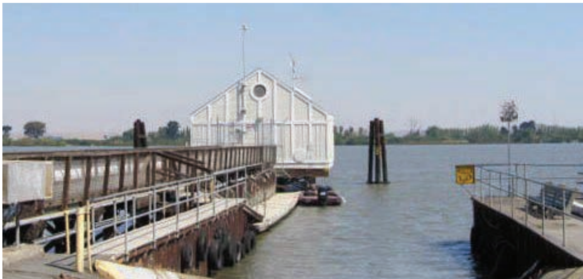
Figure C-1. River Pumping Station is constructed on pier above the San Joaquin River. The PS needs interior renovation and some improvements to the discharge pipeline.
